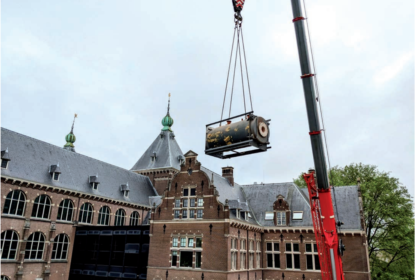
In the spring of 2023, we removed the gas boilers from our premises, making KIT the largest monument in Amsterdam to turn off the gas.
