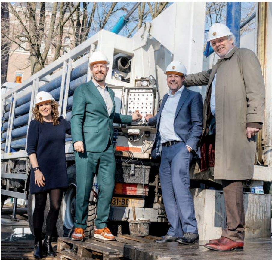
The start signal of the construction of our new underground thermal storage system (WKO), which together with heat pumps will heat our premises in the winters to come.
